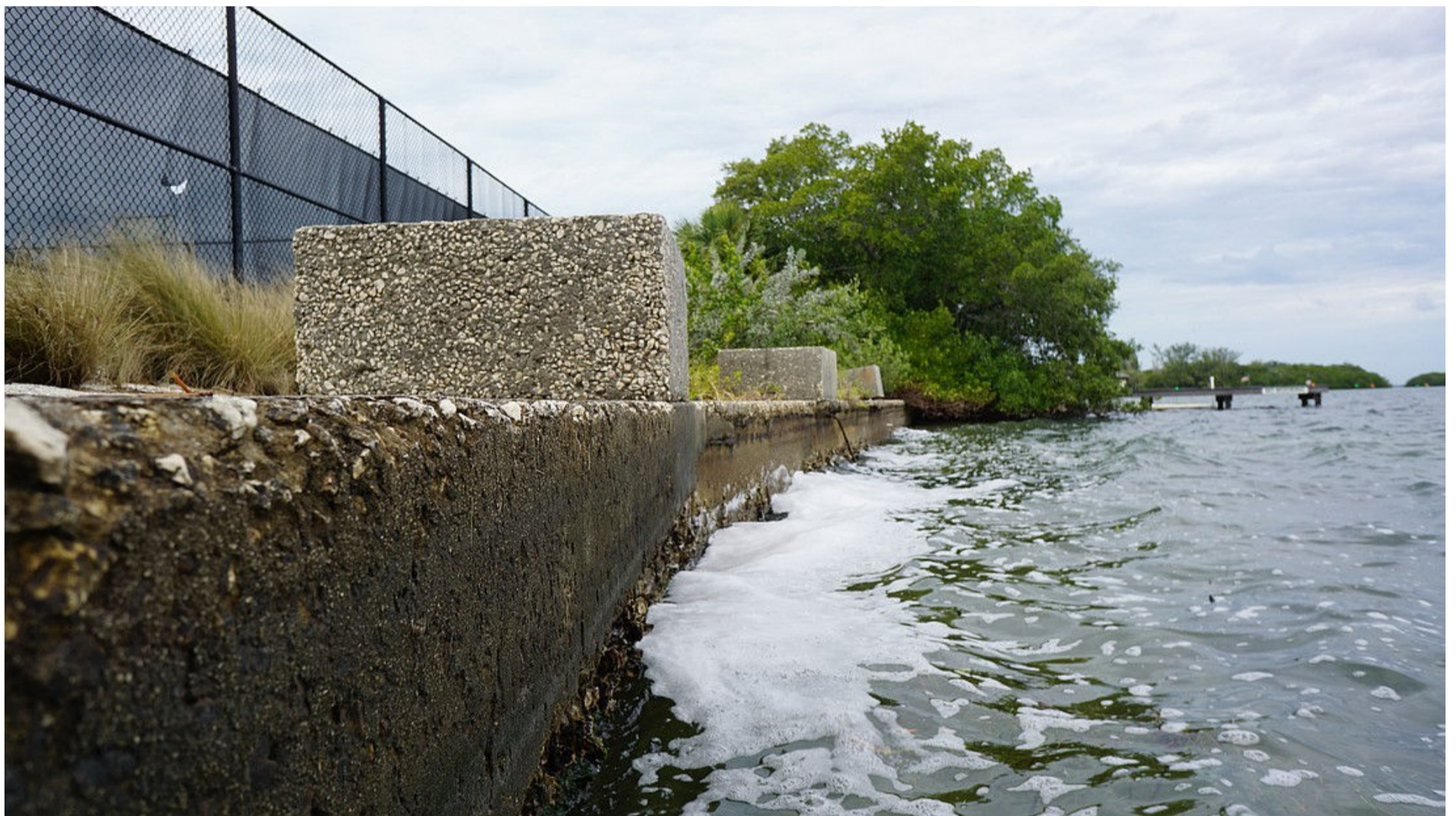
The existing concrete seawall on the north end of Bayfront Park will be replaced with a sloped living shoreline.
