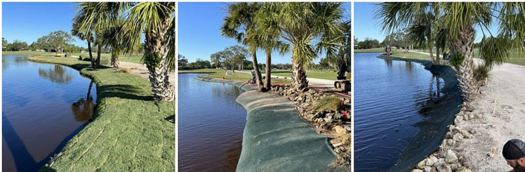
The living shoreline by International Subsea Services would implement a mesh that creates a natural-looking shoreline. Dredged sediment from the water fills the mesh covering, which has minimal impact on the surrounding area. From there, planting can occur directly on the mesh. The process is shown from right to left.
