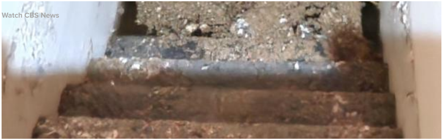
Jaime Ziadie says his home was filled with floodwater and what he calls a "green sludge" during Hurricane Ian.
